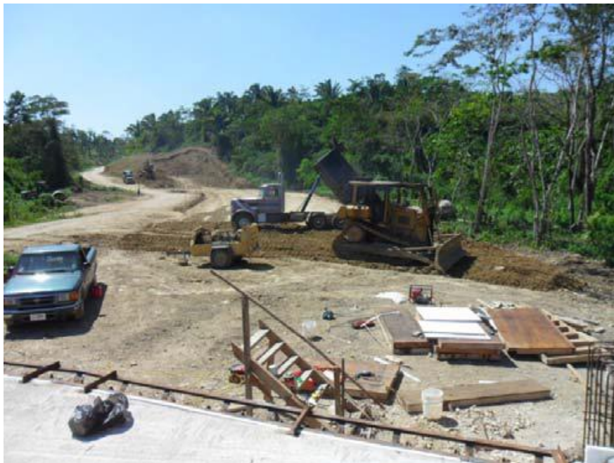
Photo 2: Cut to fill operation occurring just beyond the Rio Blanco Bridge, associated with the Rio Blanco realignment- Ch 20900m.
