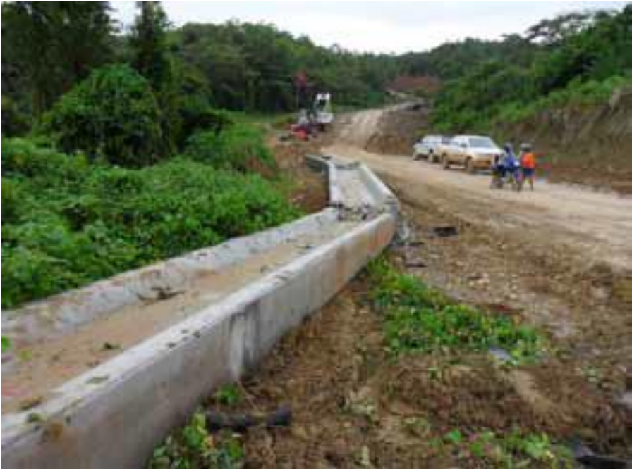
Photo 4: Broken Rio Blanco Bridge beam
