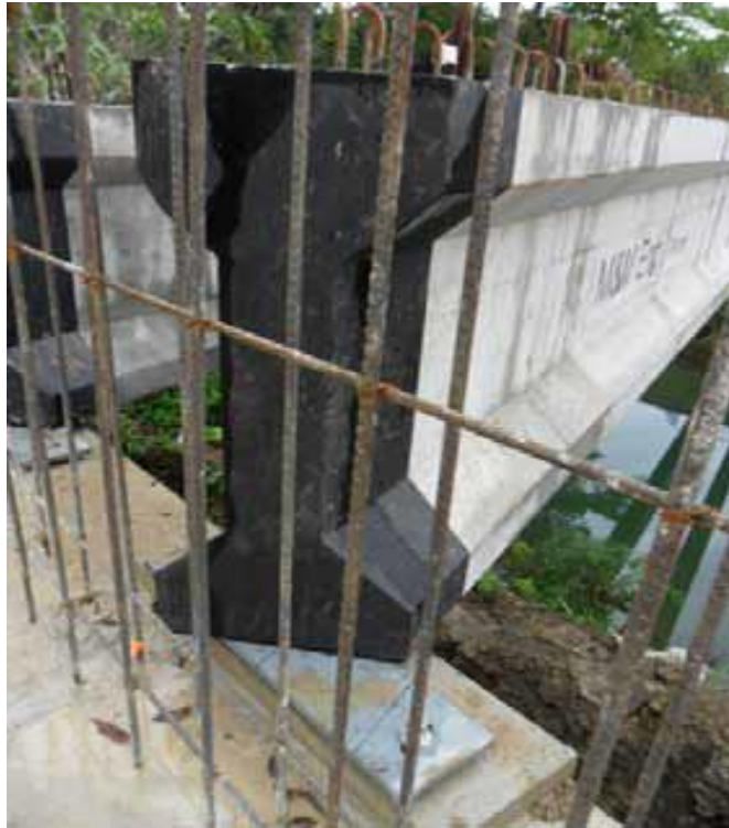
Photo 5: Placement of Rio Blanco Bridge beam showing incorrect skew that was cast into the end of the beams. Design has made amendments to beam base plants and abutment back will accommodate to construction error.
