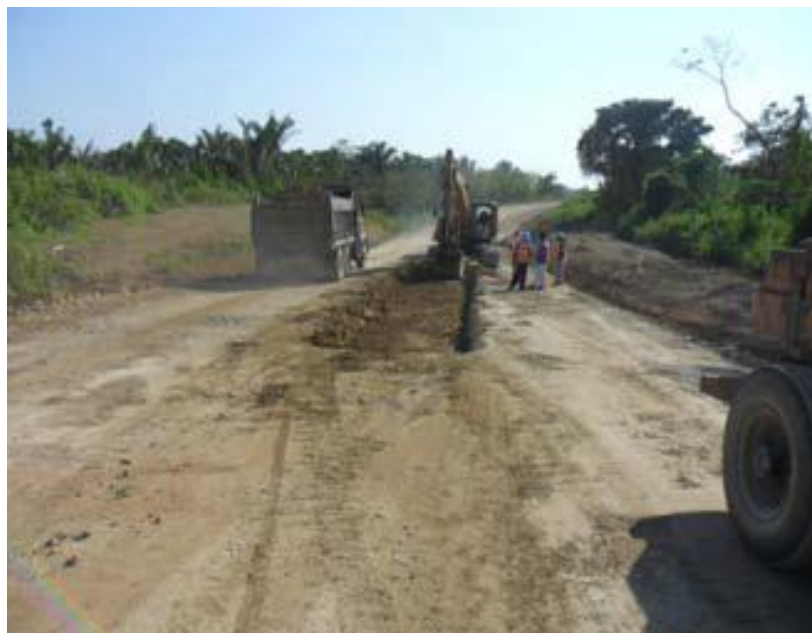
Photo 2: Undercutting wet subgrade -approx chainage 24180m – pueblo Viejo Village.
