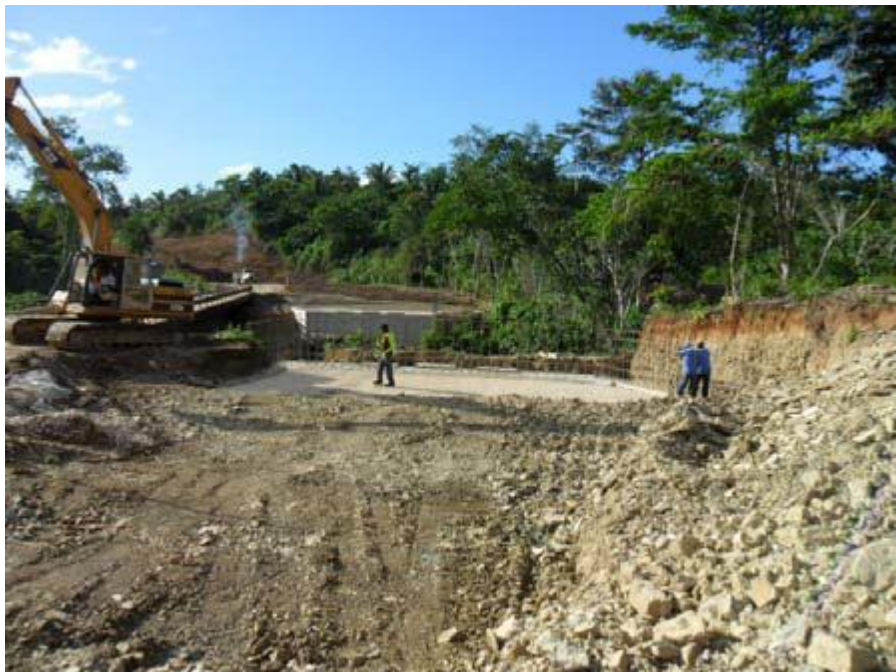
Photo 6: -Rio Blanco Bridge - Abutments cast to bearing shelf level. Area backfilled awaiting arrival of bridge beams.
